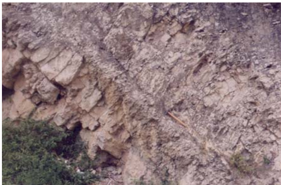
Fig. 15.5 Beds with development of cleavage and toppling of cleavage slices, a detail of Fig. 15.4. Right is to the north
