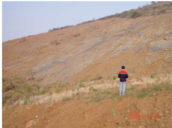
Fig. 8.5 The exposed planar sliding surface, which is also a sandstone bedding plane (there is a damaged rice paddy in front of the person)
