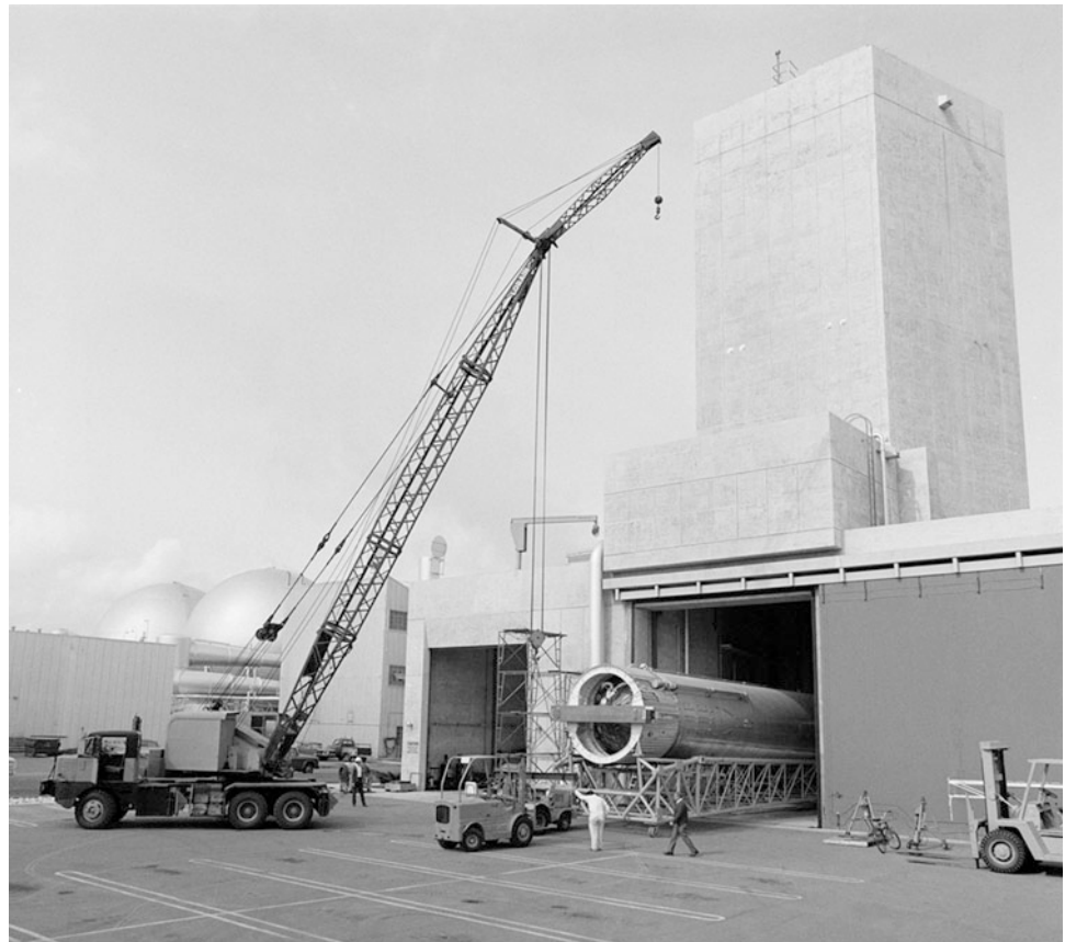
Fig. 17.9 An Atlas booster is introduced through the massive steel door ( slid to the right ) into the large airtight building which can be pumped down to vacuum or Mars pressures. The Marswit facility (Fig. 17.10) was installed in this building. Image: NASA
