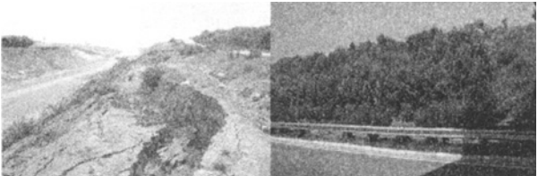
Picture 10. Comparison of cut slopes before and after treatment in the section of K136+040-K136+450
