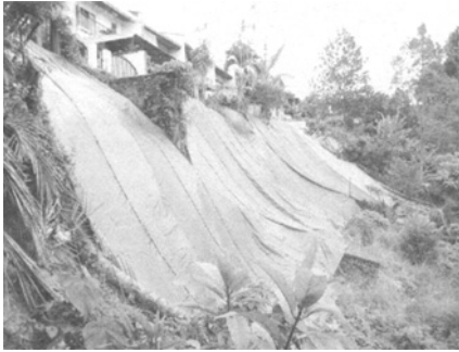
Figure 8. Condition of slope in 2004
