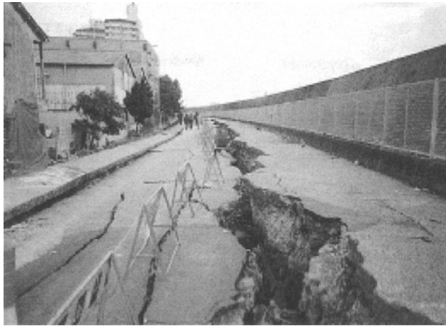
Figure 3. Seismic damage to high tide protection wall in highly industrialized area during 1995 Kobe earthquake (Kanzaki river site, Kobe, Japan)
