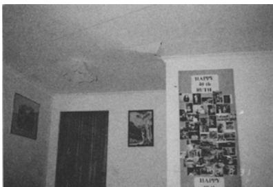
(a) crack on ceiling
