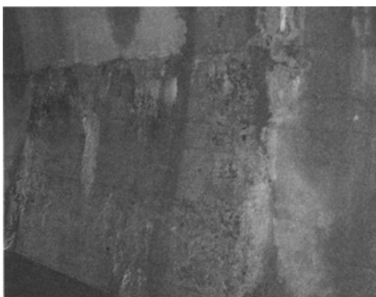
Figure 1. Deterioration of wall in the railway tunnel
