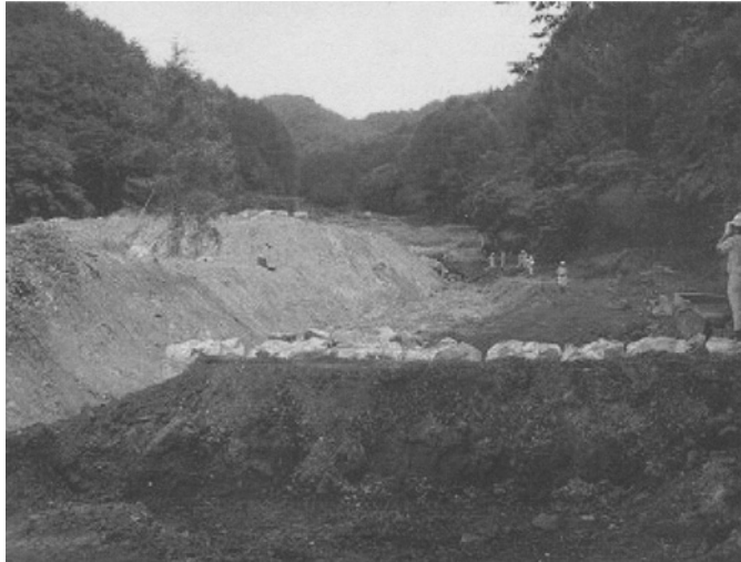
Figure 3. Scars of debris flow coming down the valley
