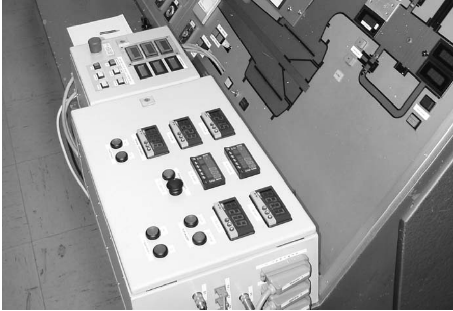
Fig. 2. Control panel for the nozzle flow integrated into the operation desk of the facility
