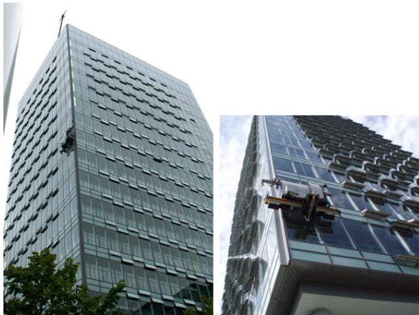
Fig. 7. SIRIUSc on the high-rise building of the Fraunhofer-Gesellschaft's headquarters in Munich
