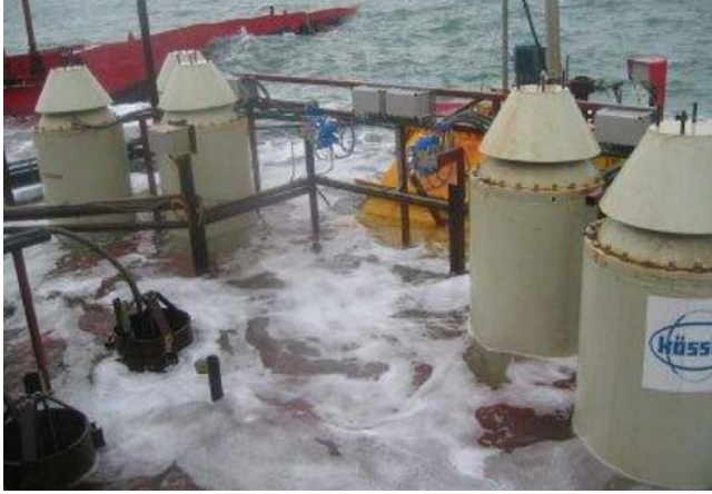
Fig. 7.80. Turbines in the reservoir of the prototype: The structure in the background is the siphon turbine, the grey towers are five of the six cylinder gate turbines, and the small devices in unpainted steel are two of the dummy turbines
