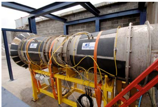
Fig. 7.44. 18.5 kW turbine-generator system
