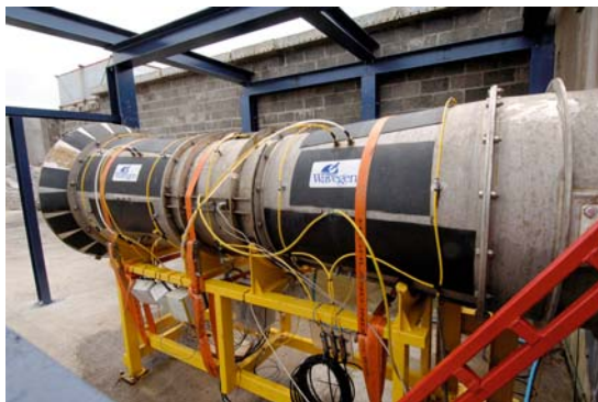
Fig. 7.44. 18.5 kW turbine-generator system
