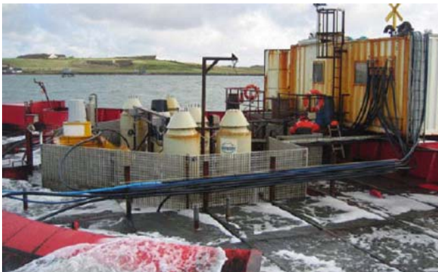
Fig. 7.81. Trash rack with 5 \times 5\text{ cm} grid openings enclosing the turbine area
