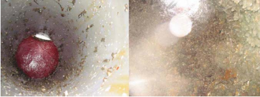
Fig. 7.82. The insides of two turbine draft tubes, on the left one painted with silicone paint, and on the right painting with conventional epoxy paint
