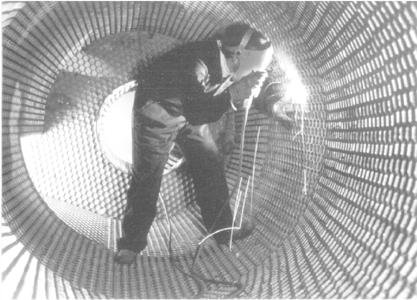
Fig. 12.1.11. 25 mm thick Hexmetal refractory anchoring grid being spot-welded to all internal surfaces of the cyclone. Note rectangular inlet chute starting in lower left-hand corner of image. Courtesy of Causeway Steel Products
