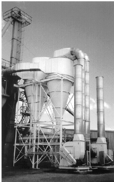
Fig. 1.3.4. A complete pull-through cyclone system for collecting various wood chips, dust and shavings including cyclones, fans and rubber-tipped rotary airlock valves. Note also outside wear plate on inlet bend. Courtesy of Koger Air Corporation
