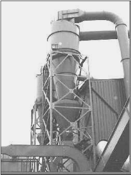
Fig. 12.1.15. Two 2.5 meter diameter industrial cyclones with 6 mm thick ceramic linings installed for erosion protection. Courtesy Omegaslate (UK) Limited
