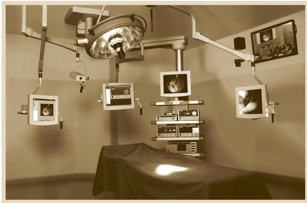
Fig. 19.10 Fully integrated operating room OR1 Karl Storz (Source: Karl Storz)
