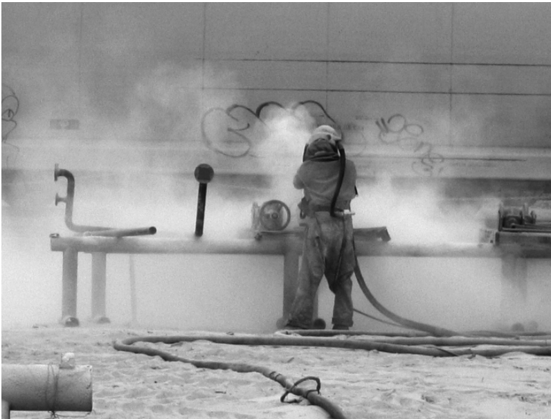
Fig. 1.3 Application of blast cleaning for the surface preparation of steel (Photograph: Muehlhan AG, Hamburg)
