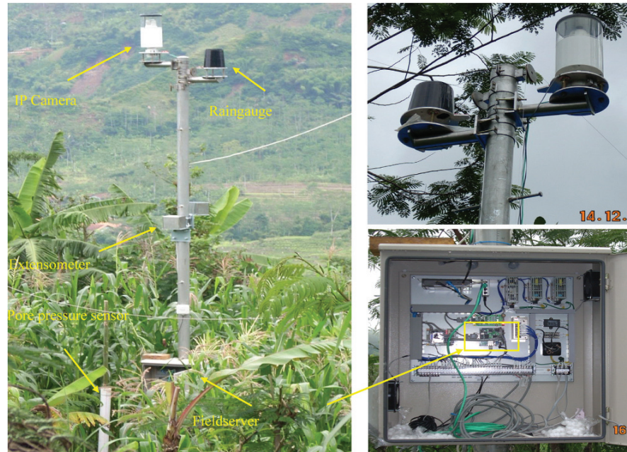
Fig. 20.7 Outdoor unit of real-time monitoring equipment
