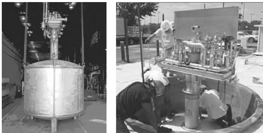
Fig. 4.7 Air products underground LH 2 tank installed at the shell hydrogen refuelling station in Washington DC in 2004
