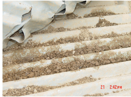
b Dry Deposits on Fills
