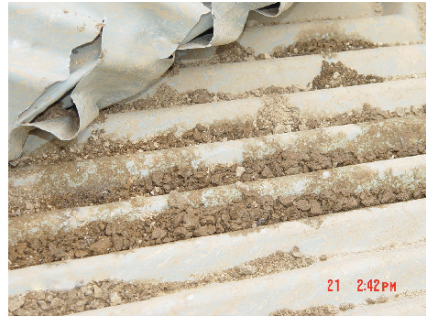
b Dry Deposits on Fills
