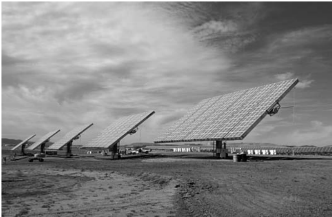
Fig. 12.6. Five HCPV systems generating power for the APS grid
