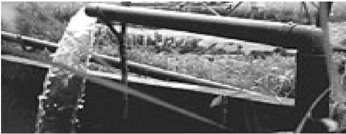
Fig. 12.8. The HCPV system can provide electrical power for water pumping
