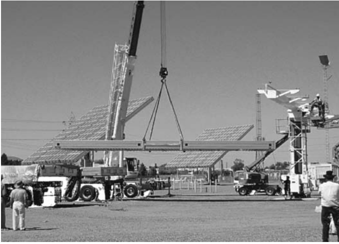
Fig. 12.17. A crane lifts the first module from the truck to the torque tube
