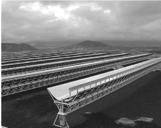
Fig. 1.11. The EUCLIDES demonstration power plant in Tenerife (1998) subsidized by the EU to industrialize the Madrid Prototype (1995). The mirrors were shaped aluminium plates covered with silvered acrylic film which cast 3.2\text{ W/cm}^2 on receivers including SATURN cells. The partners were ITER, BP Solar and UPM
