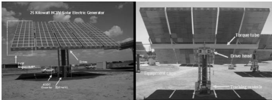
Fig. 12.10. Major subsystems and components of the Amonix HCPV system
