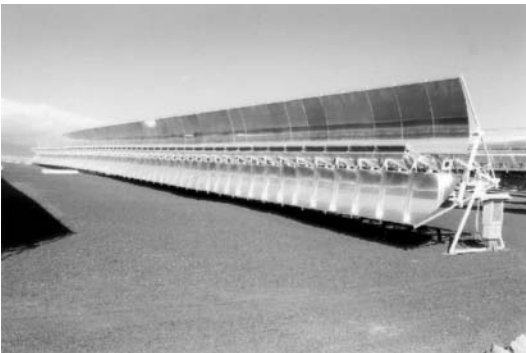
Fig. 13.13. EUCLIDES line at the Tenerife plant. Each line is 84m long and has an aperture area of 232 \text{ m}^2
