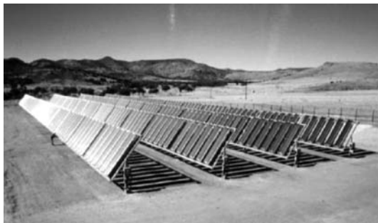
Fig. 1.9. A two-axis tracking 100-kW ENTECH power plant in Texas. System efficiency of up to 14% was demonstrated with this technology at 20 suns: curved Fresnel lenses showed optical efficiency of over 85%. Different cells were used to make the receivers
