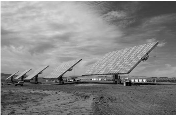
Fig. 12.6. Five HCPV systems generating power for the APS grid
