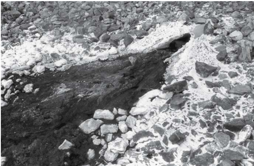
Fig. 2.17. Scalded seepage area at the base of White's waste heap (Fig. 2.16). The clay seal has cracked, and water infiltration into the dump has increased since the installation of the cover in 1984. Saline, acid seepages emanate from the base of the dump and precipitate abundant sulfate and iron oxyhydroxide efflorescences
