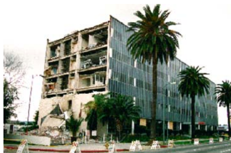
Figure 1: A building that did not suffer structural damage but the complete failure of the outer walls meant a risk of injury to pedestrians [3]
