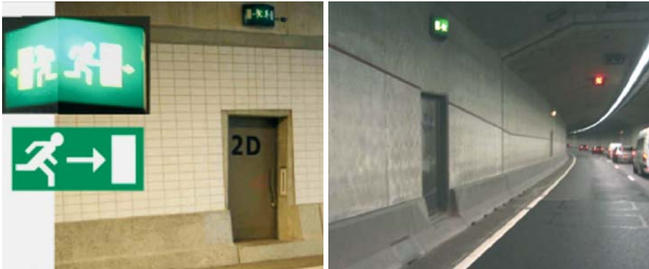
Figure 2: Marking of emergency exits with illuminated signs above the door (situation 2001 and 2004, left to right).
