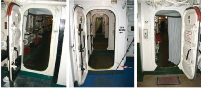
Figure 4: Components on HMS BRISTOL, a) WaterTight Door with lever, b) Airlock, c) Smoke Curtain
