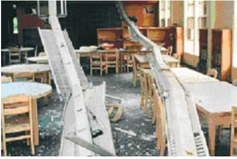
Figure 3: Damage to suspended ceiling and recessed ceiling lights [4]
