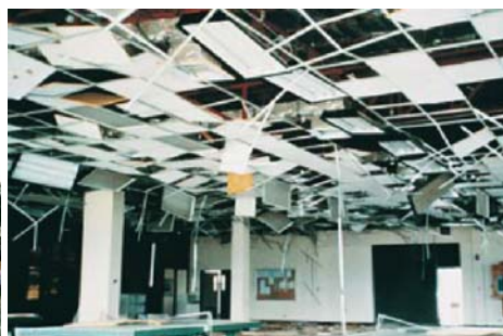
Figure 2: Failure of pendant light fixtures in a school library [4]
