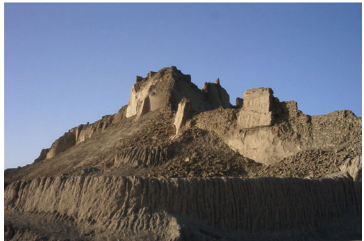
Fig. 7.7 Damage of brittle structure (Arg-e-Bam Castle after 2003 Bam earthquake, Iran)
