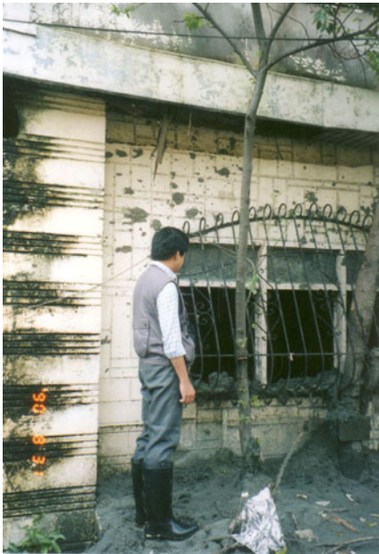
Fig. 18.4 Ejected sand on wall (Dagupan, 1990)
