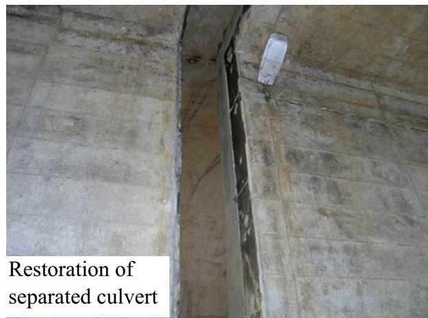
Fig. 14.5 Distortion of embedded structure due to deformation of highway embankment
