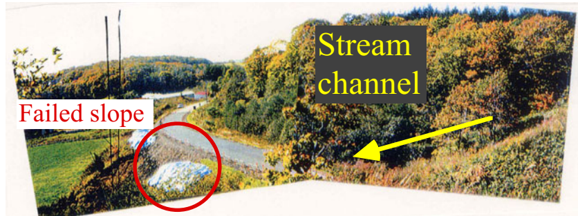
Fig. 14.6 Surface sliding of road embankment at Nakachambetsu site in 1994
