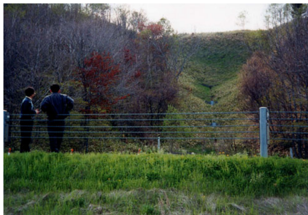
Fig. 14.44 Small creek at the place of embankment failure (Photo taken by T. Honda in May, 2000)
