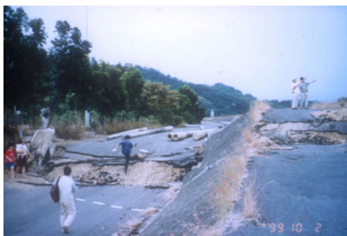
Fig. 14.2 River dike distorted by fault action at Wufeng in Taiwan
