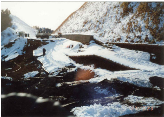
Fig. 14.43 Failed shape of Itoizawa road embankment in 1993
