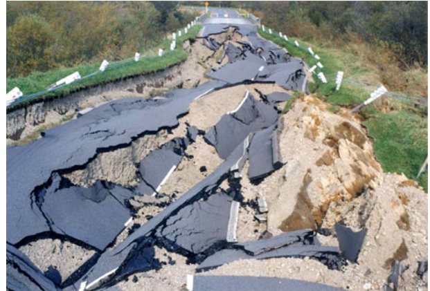
Fig. 14.12 Failure of road embankment at Chiebunnai Bridge in 1994
