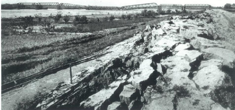
Fig. 14.14 Cracks at the top of Nagara River dike caused by 1891 Nobi earthquake (Photo supplied by Ministry of Constructiton)
