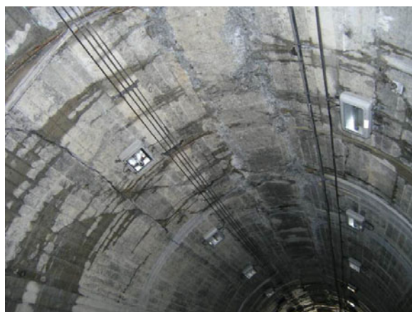
Fig. 13.25 Tension crack in top part of Haguro Tunnel
