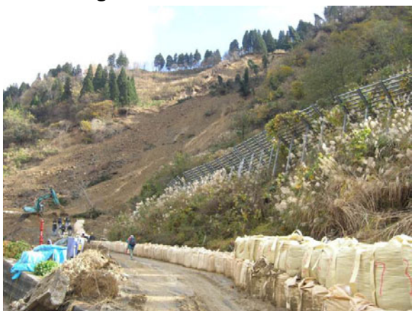
Fig. 13.26 Landslide near the western entrance of Haguro Tunnel
