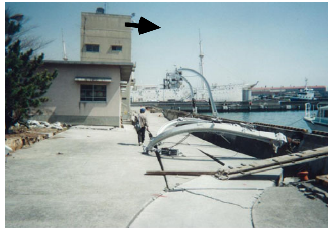
Fig. 13.18 Active seismic failure of quay wall and tilting of building behind the wall
