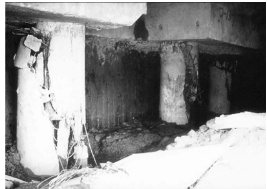
Fig. 24.7 Damage of piles caused by lateral soil flow (by Prof. K. Tokimatsu)
