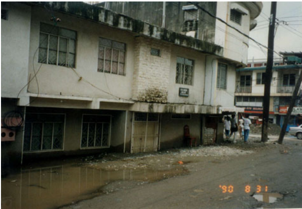
Fig. 18.40 Subsidence of building in Dagupan City due to liquefaction
