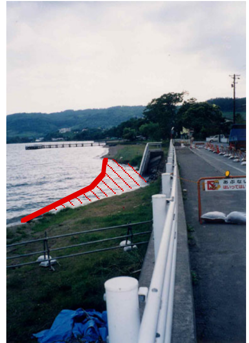
Fig. 15.54 Earthquake-induced failure of caldera wall (Tohya Lake, 1993)
