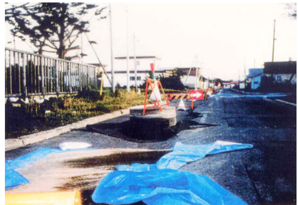
Fig. 17.18 Floating of manhole in Shibetsu
