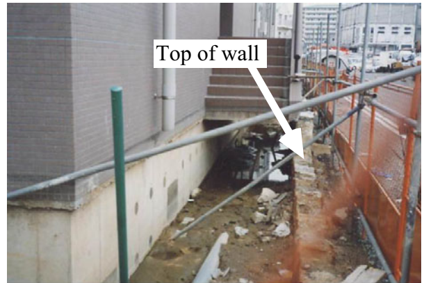
Fig. 26.11 Shimagami pumping station behind quay wall in Kobe (photograph by Prof. J. Koseki)
