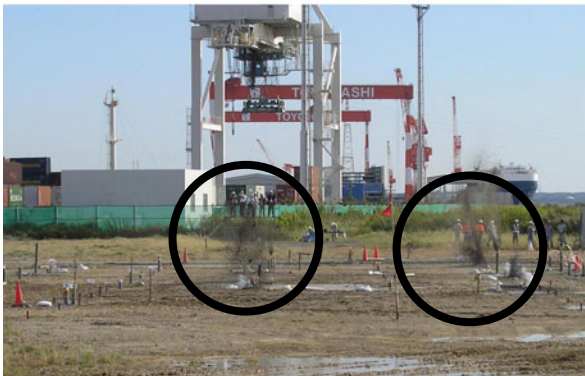
Fig. 26.141 Blasting and leaking gas from bore hole
