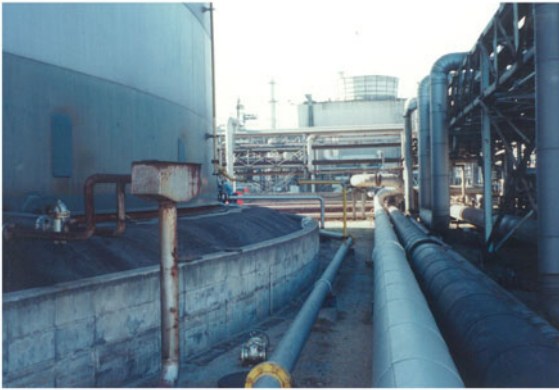
Fig. 26.24 Narrow space in oil refinery plant
