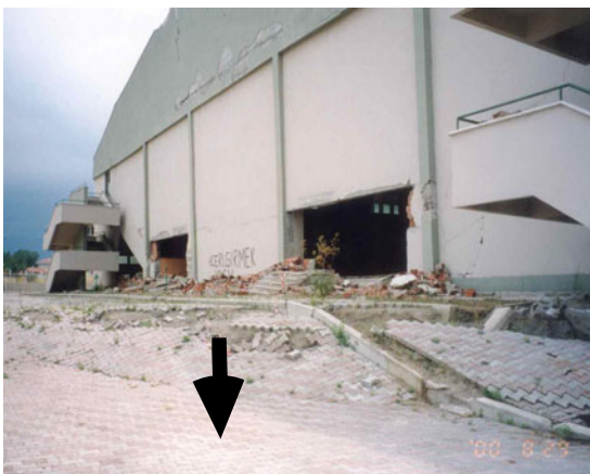
Fig. 16.47 Fault action at surface of Gölcük
