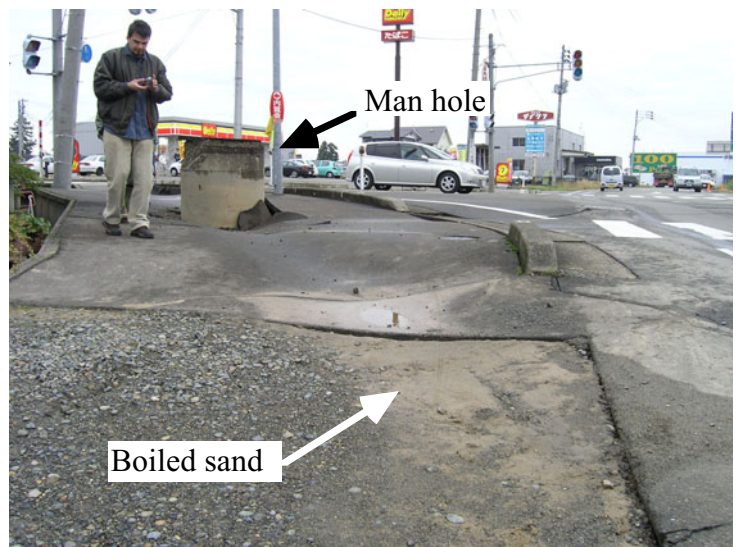
Fig. 26.137 Uplift of sewage manhole and boiled sand as evidence of backfill liquefaction (Ojiya City, 2004 Niigata Chuetsu earthquake)
