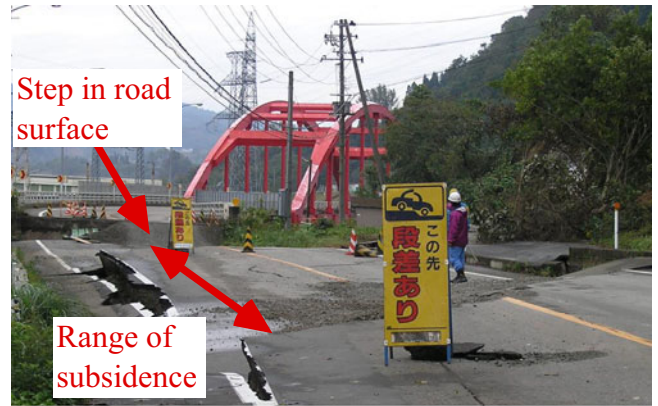
Fig. 14.16 Bridge out of service due to subsidence of approach embankment (Minami Yamabe Bridge of Ojiya City, 2004 Niigata-Chuetsu earthquake)
