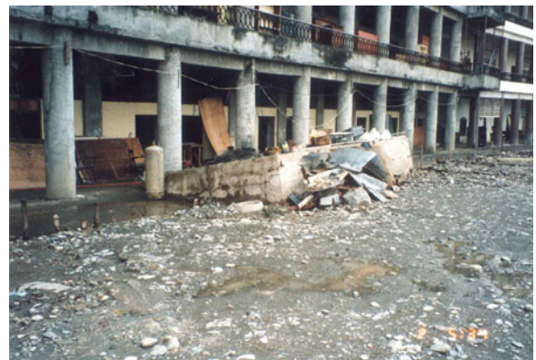
Fig. 17.16 Floating of sewage tank
