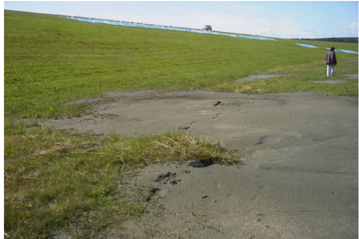
Fig. 26.3 Minor distortion in Tokachi-river dike in 2004 caused by minor liquefaction
