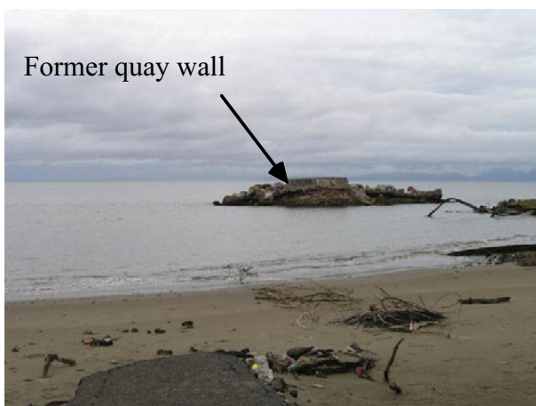
Fig. 16.62 Former quay wall and eroded backfill area (Banda Aceh, Indonesia)
