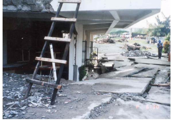
Fig. 17.3 Subsidence of building in Dagupan City
