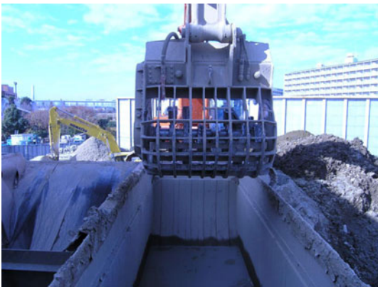
Fig. 26.139 Production factory for mixing waste soil with cement, gravel, and water
