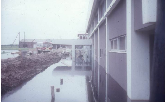
Fig. 25.57 Terminal building of Niigata Airport after liquefaction and subsidence (Department of Civil Engineering, University of Tokyo)
