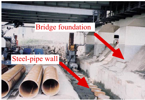
Fig. 26.17 Installation of steel-pipe wall for protection of bridge foundation from lateral soil movement (Photo by Prof. S. Yasuda)
