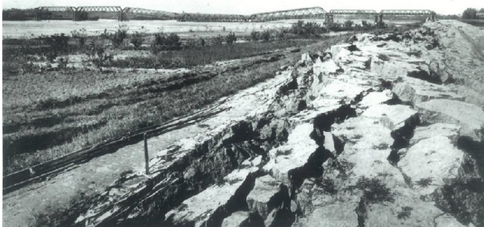
Fig. 14.14 Cracks at the top of Nagara River dike caused by 1891 Nobi earthquake (Photo supplied by Ministry of Construciton)
