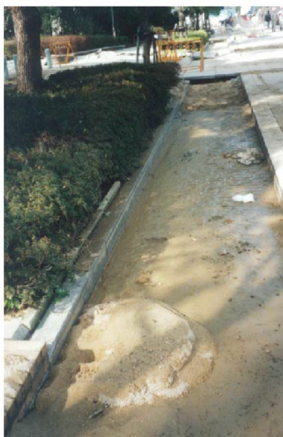
Fig. 18.44 Minor liquefaction in Higashi Park on inland side of original coast line in Kobe
