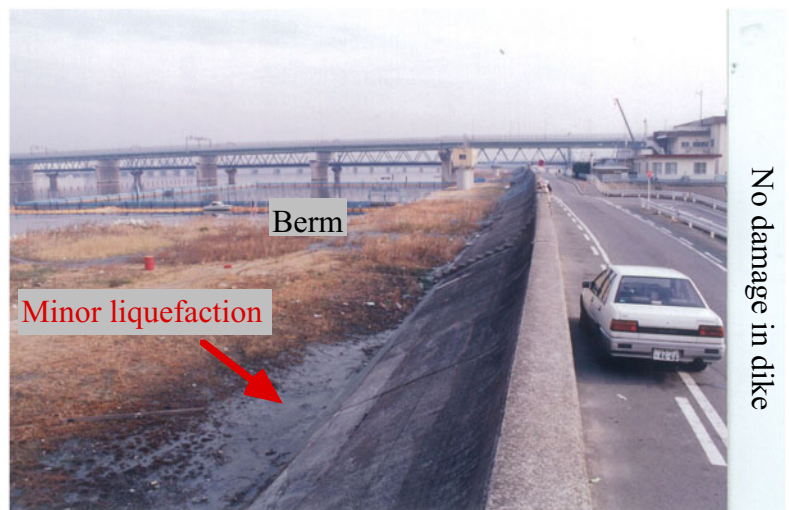
Fig. 26.12 Undamaged dike of Yodo River at Takami site in Osaka (supplied by MLIT, Government of Japan)
