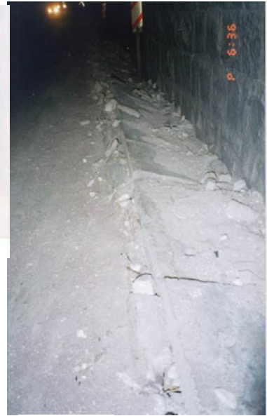
Fig. 16.33 Distortion of cover stone of drainage trench due to reduced width (Manjil earthquake)
