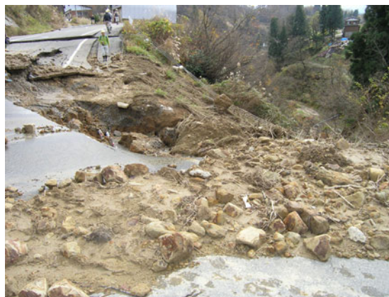
Fig. 14.9 Failure of road embankment during the 2004 Niigata-Chuetsu earthquake
