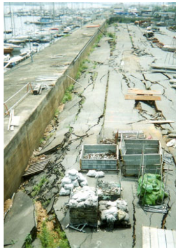
Fig. 24.6 Tensile deformation at surface of backfill soil (Nishinomiya Harbor in 1995)
