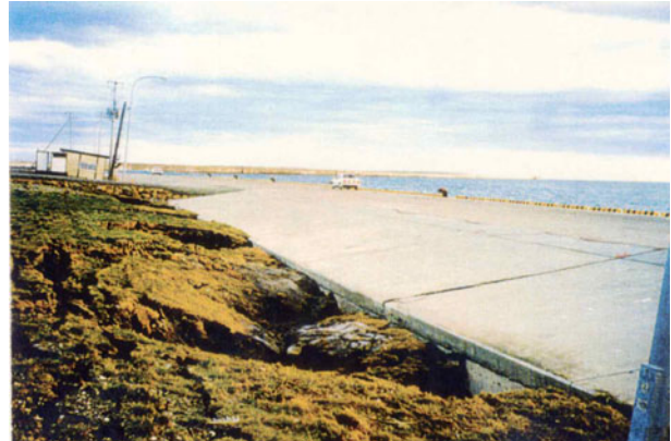
Fig. 17.21 Liquefaction damage at Hanasaki
