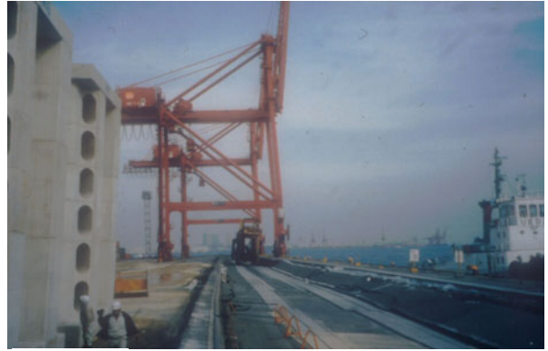
Fig. 24.5 Lateral displacement of caisson quay wall in Port Island, Kobe, in 1995
