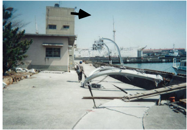
Fig. 13.18 Active seismic failure of quay wall and tilting of building behind the wall
