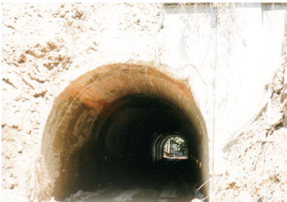
Fig. 16.36 Compressed arch of tunnel in Taiwan (1999)
