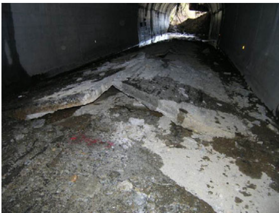
Fig. 13.24 Distorted shape and buckling of pavement in Haguro Tunnel, Niigata-Chuetsu
