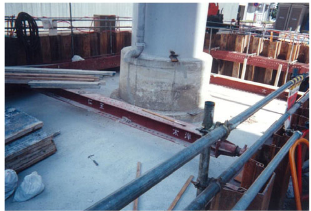
Fig. 24.66 Increasing lateral resistance of pile foundation by enlargement of pile cap and increasing number of piles (in the center of Sunnomiya, Kobe)
