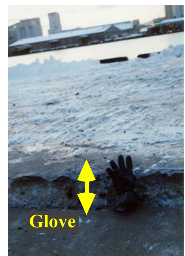
Fig. 26.89 Subsidence of ground with gravel drains relative to stable quay wall (Kushiro Harbor, 1993)
