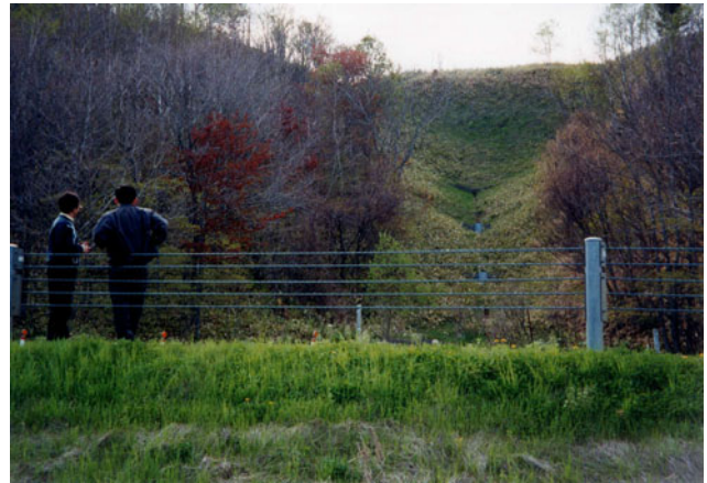
Fig. 14.44 Small creek at the place of embankment failure (Photo taken by T. Honda in May, 2000)
