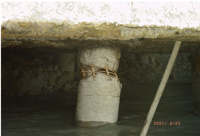
Fig. 13.28 Damaged pile in Navrakhi Harbor, Gujarat Province, India, in 2001
