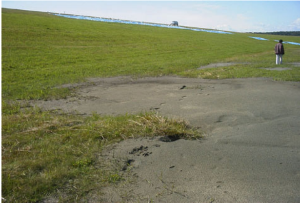
Fig. 17.13 Minor liquefaction near Tokachi River dike in 2003
