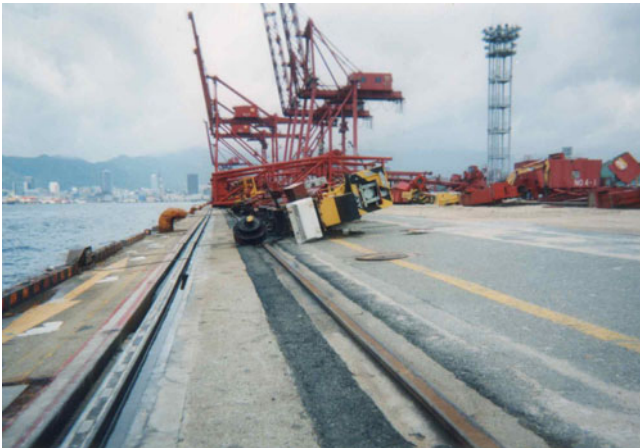
Fig. 24.33 Distortion of caisson quay wall in Kobe
