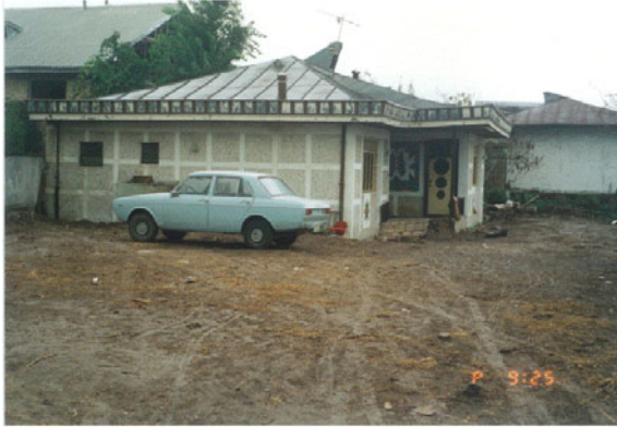
Fig. 17.58 Liquefaction under private house (Gilan, Iran in 1990)
