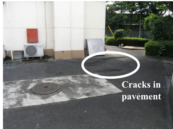
Fig. 9.41 Differential settlement around building
