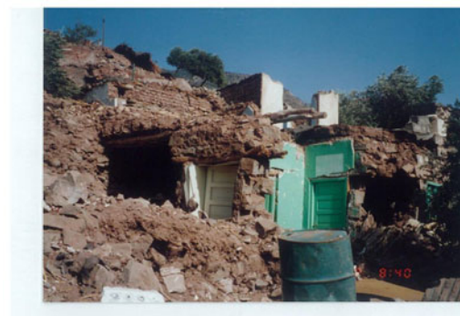
Fig. 5.37 Collapse of adobe house with heavy roof (Gilan, Iran, 1990)
