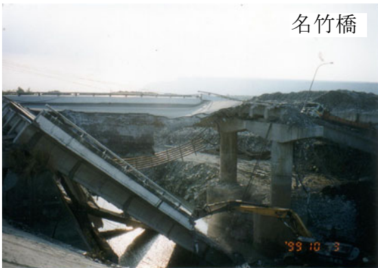
Fig. 14.21 Total collapse of road bridge in Taiwan, 1999 (after 1999 ChiChi earthquake in Taiwan)
