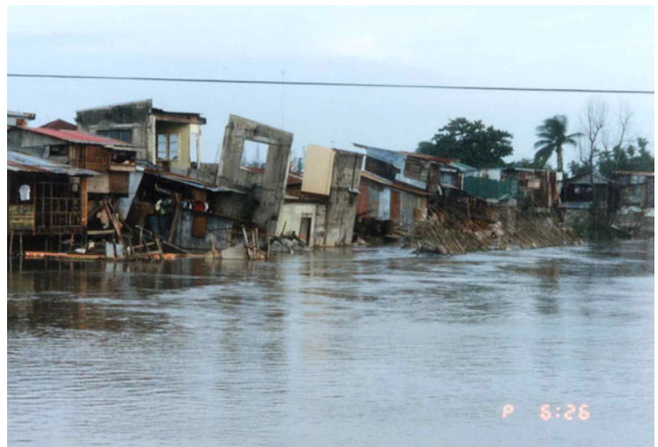
Fig. 17.23 Lateral movement of embankment in Dagupan
