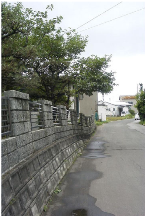
Fig. 17.60 Distortion of retaining wall due to subsurface liquefaction (Noshiro City in Akita, Japan)
