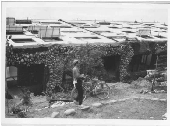
Fig. 17.7 Base of Kawagishi-cho apartment building after falling (Department of Civil Engineering, University of Tokyo)
