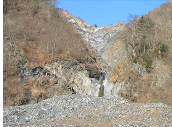
Fig. 15.10 Unstable mountain slope
