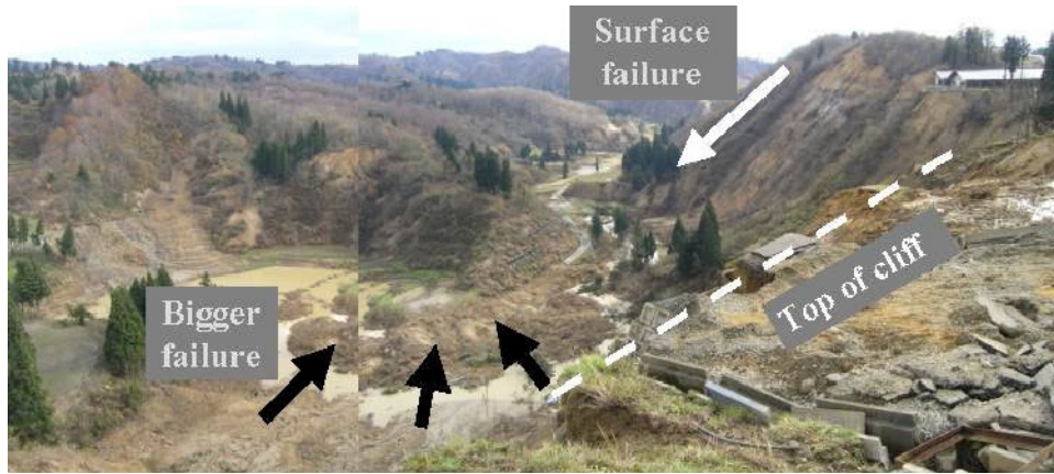
Fig. 15.43 Different extents of lateral movement of debris due to different volumes at Naraki after 2004 Chuetsu earthquake
