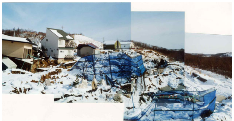
Fig. 14.7 Failure of residential development site in Kayanuma in 1993
