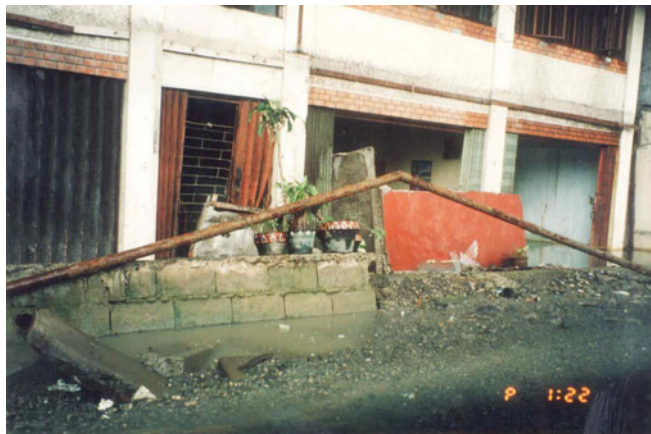
Fig. 17.24 Buckling of buried pipe in Dagupan City, the Philippines
