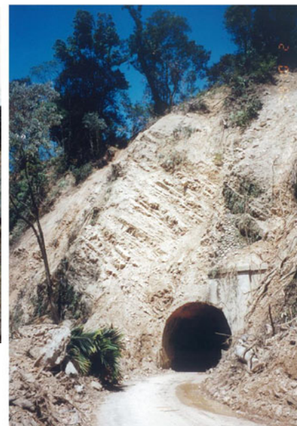
Fig. 13.23 Slope failure at the entrance of tunnel (五龍隧道 Taiwan, 1999)
