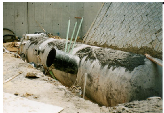
Fig. 24.13 Static liquefaction of backfill and flotation of underground fuel-storage tank
