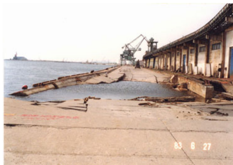
Fig. 24.8 Substantial damage of sheet-pile wall at Akita Harbor in 1983 (by Dr. K. Wakamatsu)
