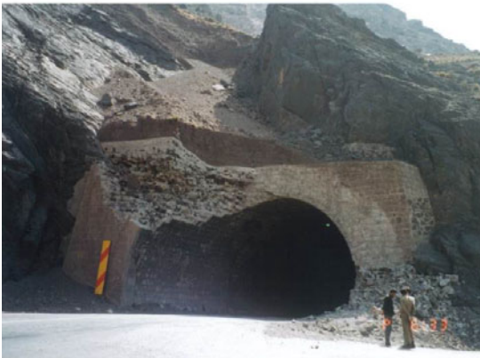
Fig. 16.34 Damage at entrance of tunnel (Manjil earthquake)
