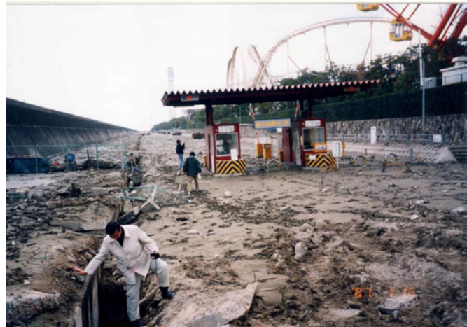
Fig. 20.9 Liquefaction of gravelly ground
