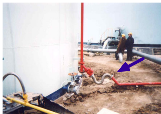
Fig. 17.33 Flexible joint of oil storage tank that absorbed heavily subsidence of tank
