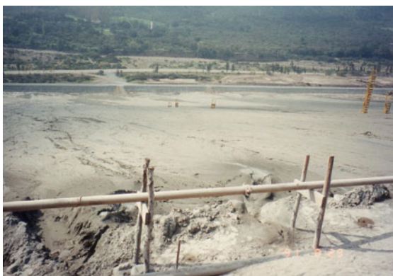
Fig. 20.22 Discharging coarse material onto downstream slope of tailing dam (Lomeral in Chile)
