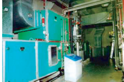
Fig. 8.69. An application of fuzzy logic in the A/C system of a large hospital in Germany saved more than 25% on energy costs
