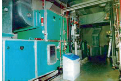
Fig. 8.69. An application of fuzzy logic in the A/C system of a large hospital in Germany saved more than 25% on energy costs
