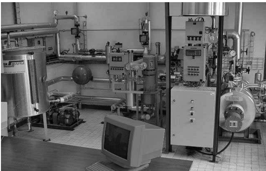
Fig. 10.49. General view of the steam generator
