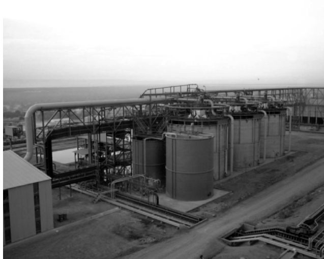
Fig. 2.4. Bioleach tanks (Bioco reactors) at the Kasese Cobalt Company (KCC) plant
