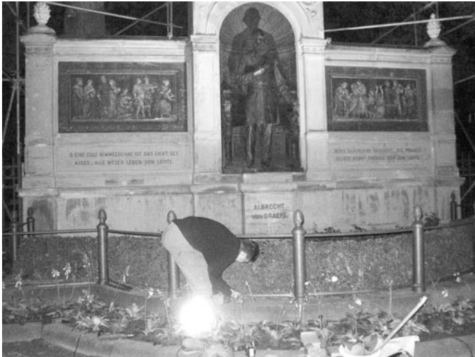
Fig. 1.7.7 Risky activity: a scene from everyday life. The author took this picture in Berlin, Germany, during a large ophthalmology conference in 2005. The worker was repairing a metallic fence: hammering, chiseling, welding, and using power tools to cut and strip. He did not wear eye protection. The sad irony of the scene is that it occurred at the memorial of Albrecht von Graefe
