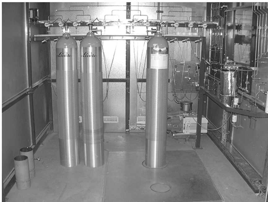
Illustration P5.1.1.1-2: View in a filling cabinet.
