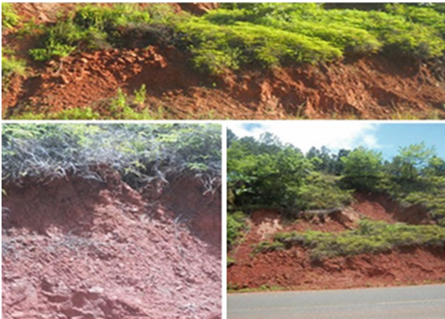
Fig. 1 Slope failure at R523 road
