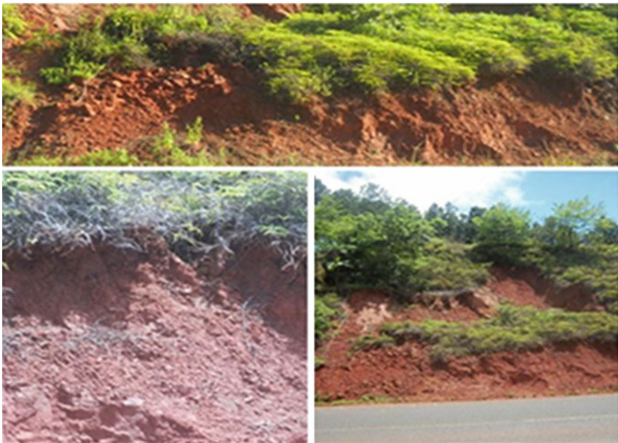
Fig. 1 Slope failure at R523 road
