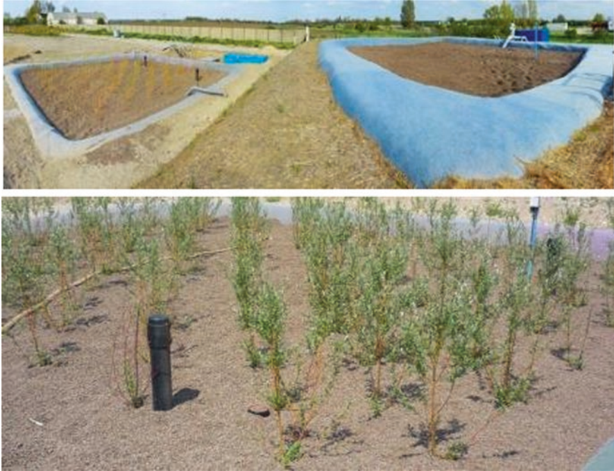
Fig. 6.3 Full-scale vertical flow constructed wetland treating contaminated groundwater in Leuna
