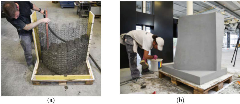
Fig. 1. (a) Concreting process of a Mesh Mould wall using a pump and (b) Finishing the wall [4]
