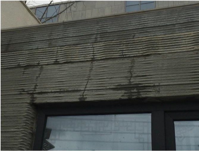
Fig. 1. Signs of local capillary suction at the interfaces between layers of printed concrete as well as at cracks, photo by V. Mechtcherine.
