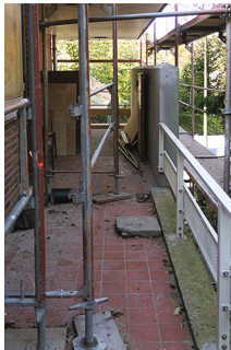
Fig. 10. Terrace along the kitchen and entrance with a view on the restored railing
