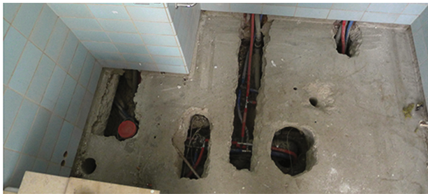
Fig. 7. New pipework from different rooms is bundled under the bathroom floor, where the contemporary vinyl finish is replaced. (© Steven van der Goes)
