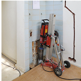
Fig. 6. Drilling installation holes through the bunker roof in one of the bedrooms
