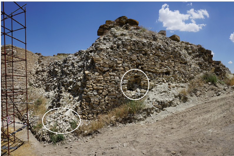
Fig. 4. Spalls of 2015 winter highlighted with circles and the MP Wall stones resting precariously above
