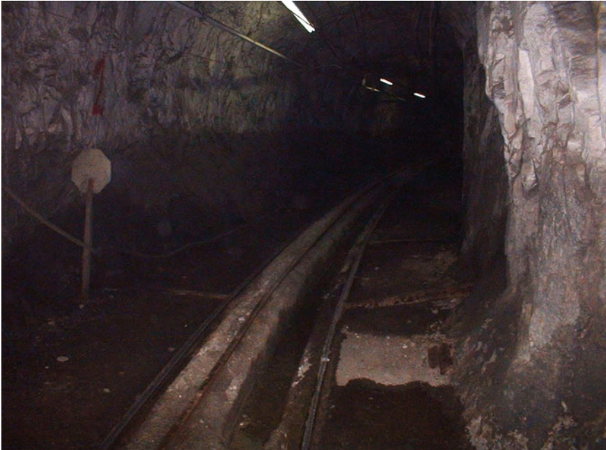
Fig. 1 Typical underground track conditions. Note the timber sprags supporting the rail against the sidewall and the material between the tracks
