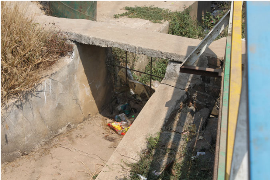
Fig. 6.3 Waste beginning to pile up against a drainage canal grate (Photo by Graham Reeder)
