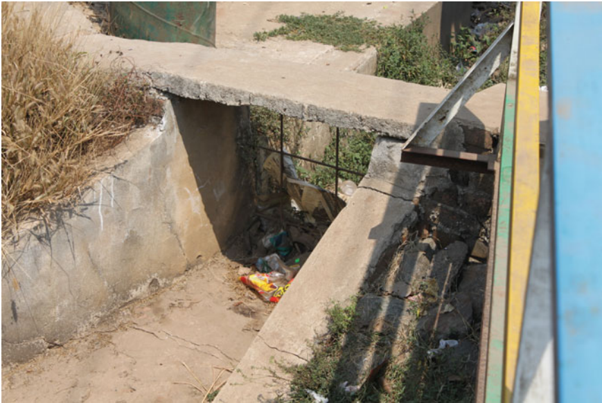
Fig. 6.3 Waste beginning to pile up against a drainage canal grate (Photo by Graham Reeder)
