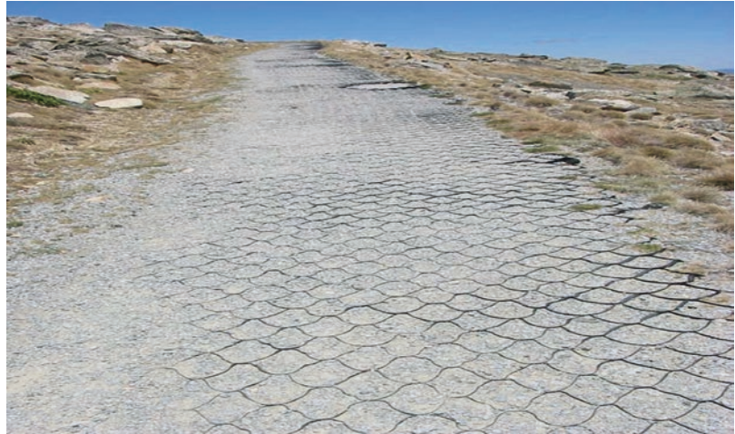
Fig. 2.6 Geotextile. Originally covered with aggregate, but this has been eroded as the geotextile was not laid deep enough so that there was an adequate aggregate fill. It should have trapped sediment and slowed surface runoff (Three Peaks project). Photo by David Huddart
