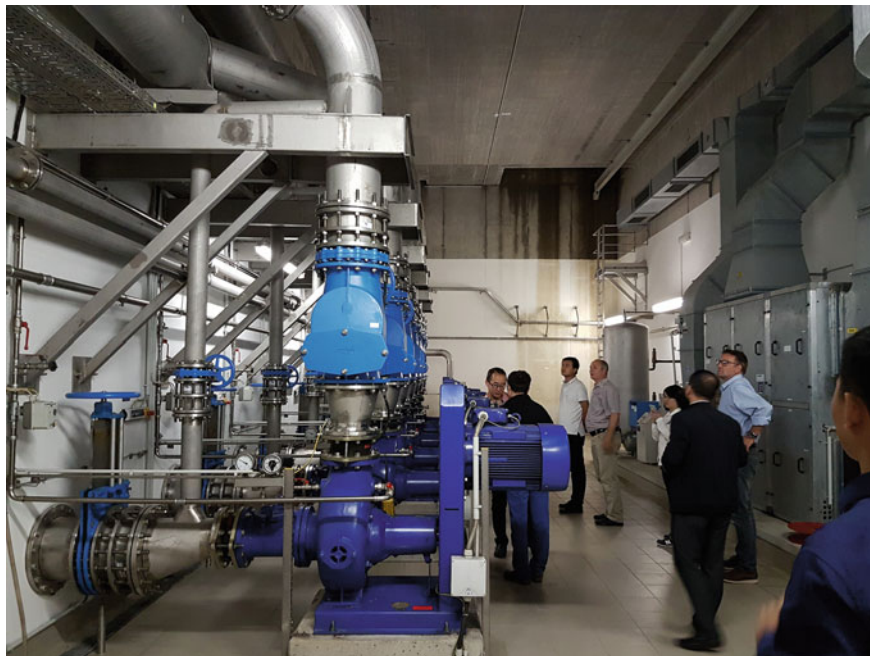
Fig. 2.34 View into the machine hall of the sewage treatment plant Kaditz (Source: UC Project)
