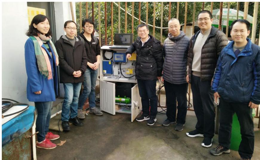
Fig. 2.38 The online monitoring stations were successfully installed in Shanghai (Source: Tongji University)
