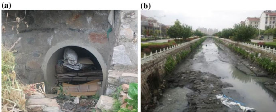
Fig. 3.3 Example of blocked sewer (a) and channelized river. (b) with sediments
