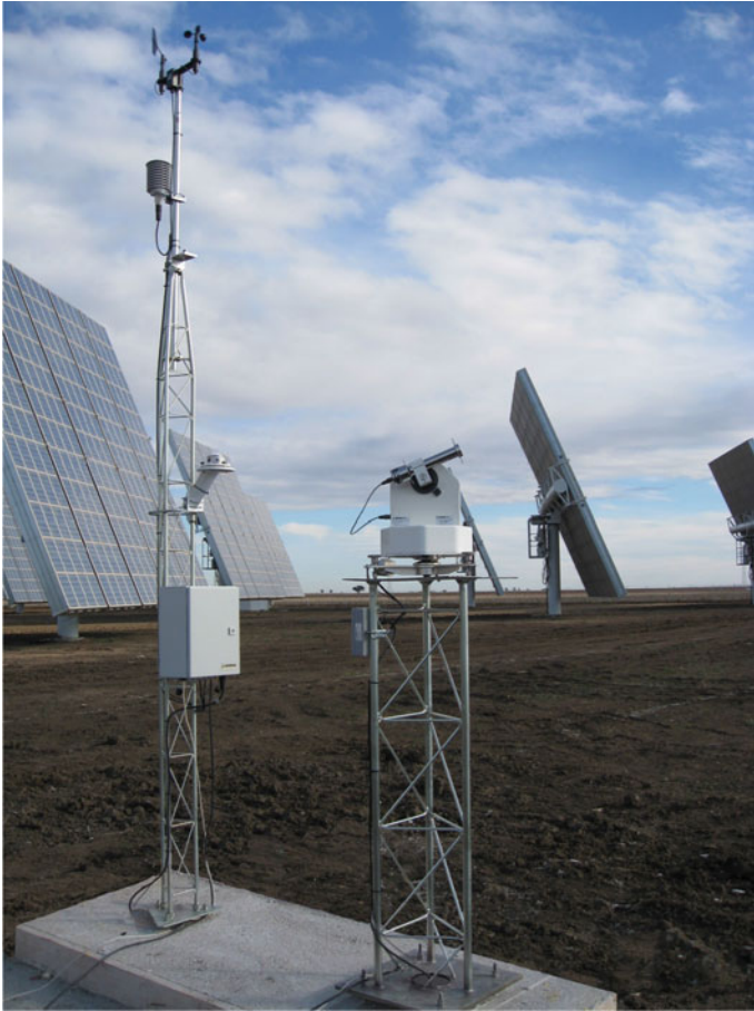
Fig. 19 Sunpower system real-time monitoring at CPV plant. Courtesy of Geonica ©
