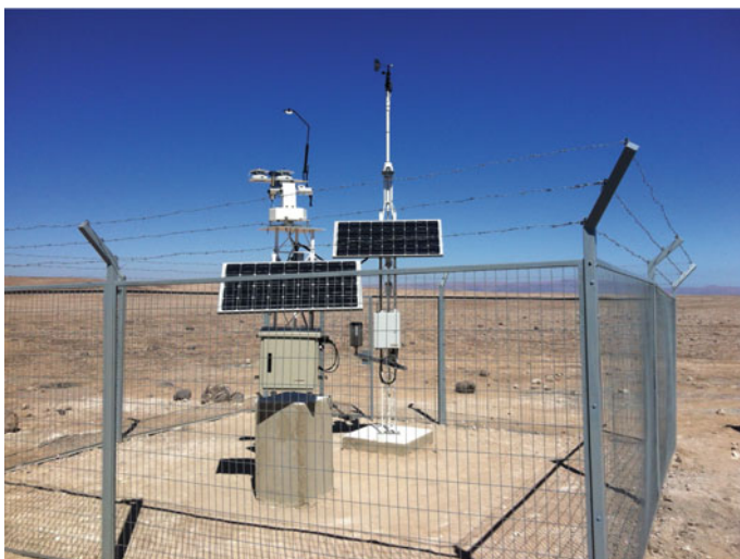
Fig. 18 Detailed view of a radiometric (from) and meteorological station (back) in a remote location working autonomously with power supplied from two PV panels. Courtesy of Geonica ©
