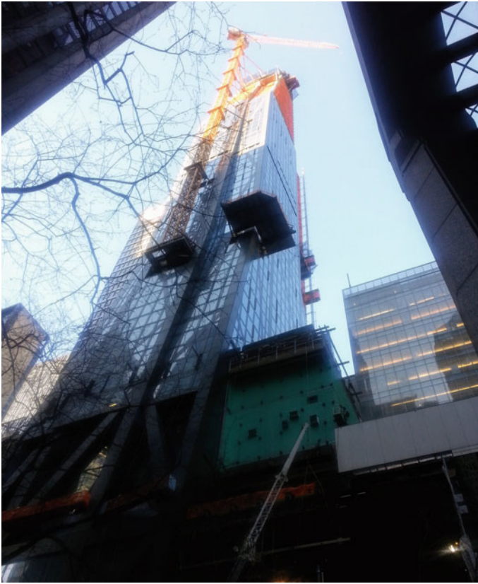
Fig. 28.11 Construction site for new MoMA building at 53W.53 in New York City. (Photograph by Tula Giannini, February 27, 2018)
