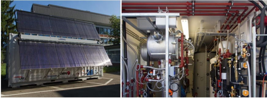
Fig. 2 Pictures of the TES pilot system with NaOH/water [1]
