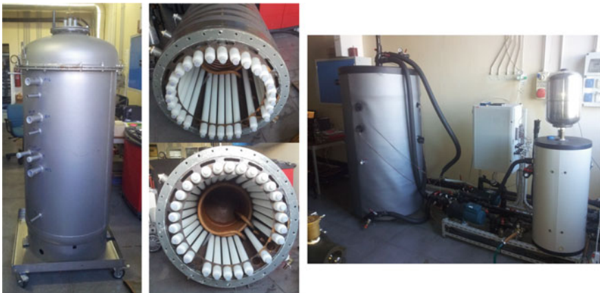
Fig. 18 Some pictures of the installed storage in the CNR-ITAE lab
