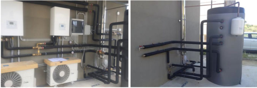
Fig. 11 Particular of the heat pumps, of the correspondent external units and of the vertical storage tank of the demonstrative smart air-conditioning plant
