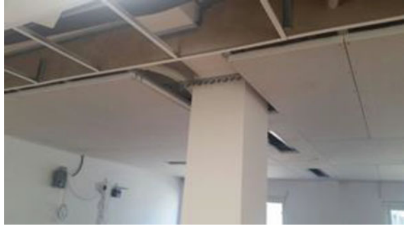
Fig. 12 Particular of the installed decoupled radiant ceilings in mineral fibre
