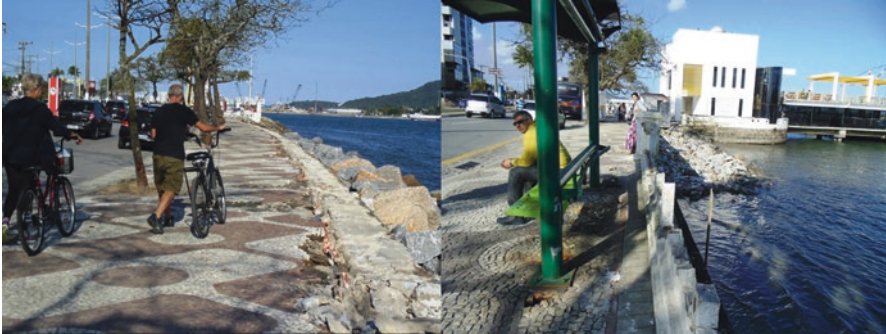
Fig. 15.4 Damages caused by intense storm surge in the city of Santos. Both pictures illustrate the destruction of the Santos walls on a part of the beach that have been suffering erosion, and it have been intensified with current climatic variations. (Photo: Danielle Almeida de Carvalho)
