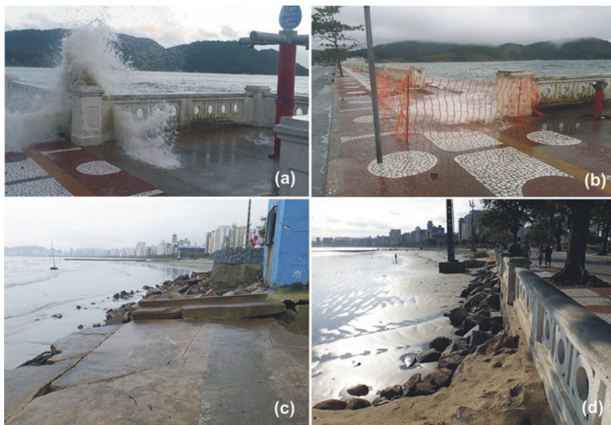
Fig. 6.2 Some impacts caused by storm surges on 07/04/2015 (a), 06/08/2016 (b), 16-08/2017 (c) and 20/05/2018 (d) in Ponta da Praia region (Southeast Zone) (photos from the first author)
