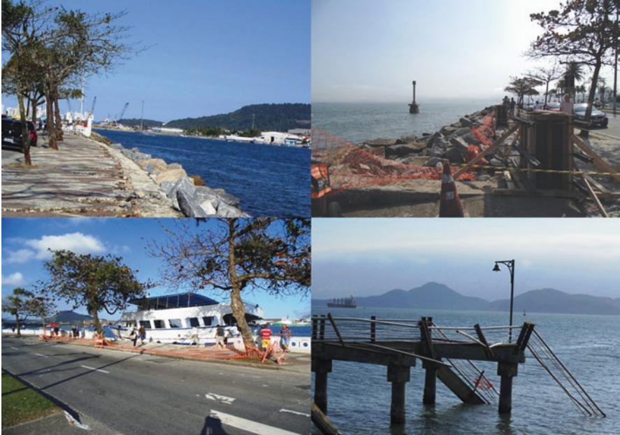
Fig. 15.6 Infrastructure damages caused by the intense storm surge event on 21 August 2016 at Ponta da Praia, Santos. (Photos Danielle Almeida de Carvalho)
