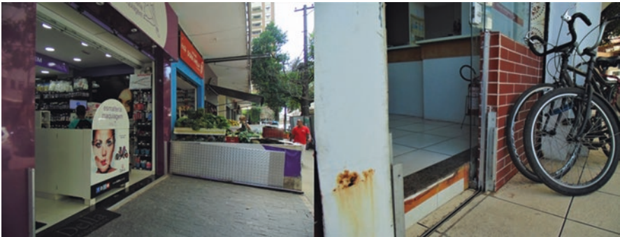
Fig. 15.7 Examples of a watergates-floodgate built by local trade owners of a cosmetics store (left) and a restaurant to prevent water intrusion in the property located at Ponta da Praia, Santos (2016). (Photos Danielle Almeida de Carvalho)
