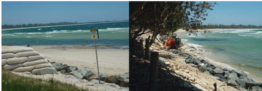
Fig. 15.1 Sandbags (left picture) and reconstruction works (right picture) in response to accelerated beach erosion in Kingscliff, New South Wales /Australia, 2011. (Photo Débora M. De Freitas)
