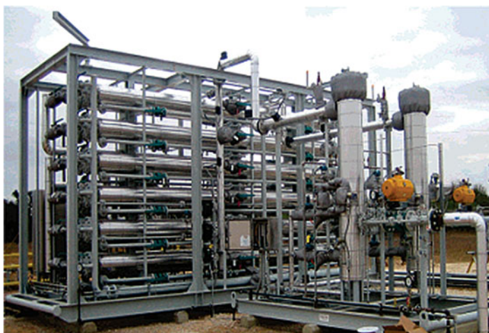
Fig. 8 Photograph of a CO 2 separation plant. (Reprinted from [7] with permission from Elsevier)
