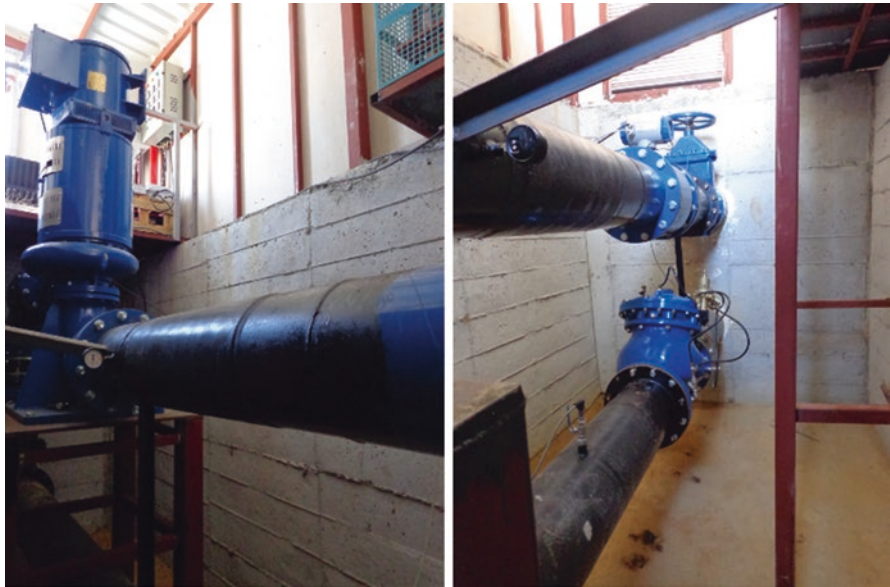
Fig. 6 Photographs of the installed PAT system [7]
