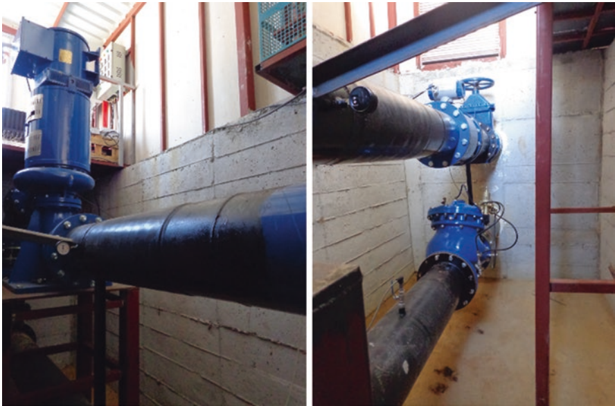
Fig. 6 Photographs of the installed PAT system [7]
