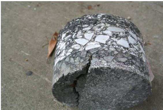
Fig. 3. High-scaling transverse reflective crack
