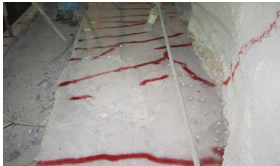
Fig. 3. Transverse cracks of downstream rock-anchored beam at 0 + 48.00
